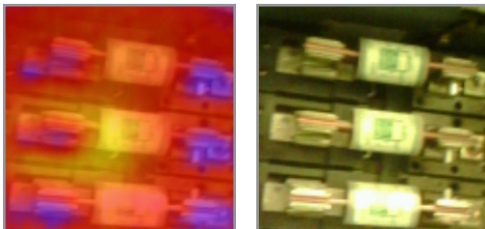
Detect issues with switchgears
